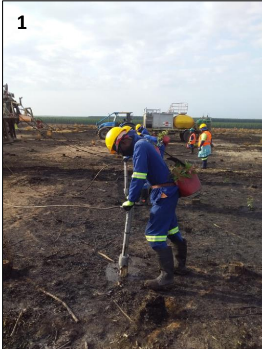
Pitting using water pressure
